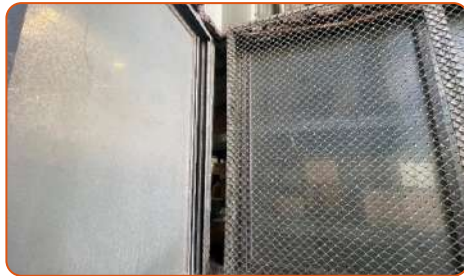
Current Condition: Damaged corrugated metal panel outside the Maintenance Section 1 workshop of Building A at the Xinying Factory.
