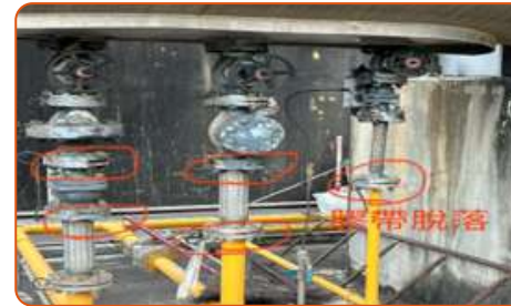
Current Condition: Sealant tape detached from the side of the high-pressure gas storage tank.
