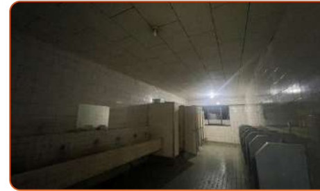
Current Condition: Lighting failure in the restroom of Building F at the Xinying Factory.
