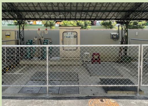
Sewage Treatment Facility at Xinying Factory
